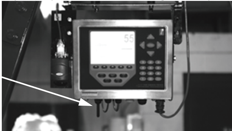
Figure 3. Location of the WLAN Antenna
